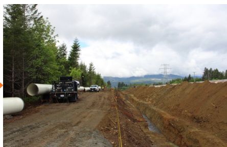
Pipe ready to be installed alongside the existing BC Hydro penstocks. (May 2020)
