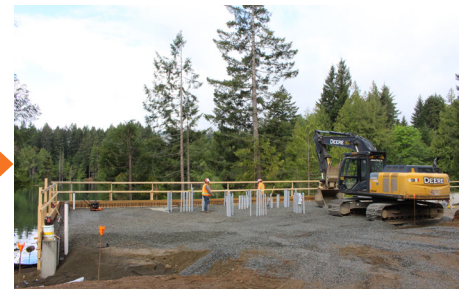
The foundation area was backfilled in preparation for the base slab to be poured. (May 2020)
