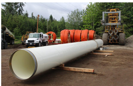
Steel pipe arrived – it will move water from the treatment plant to the existing distribution system. (May 2020)
