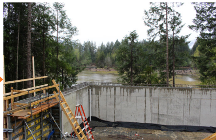
Concrete for the foundation wall of the electrical building was poured. (Apr. 2020)
